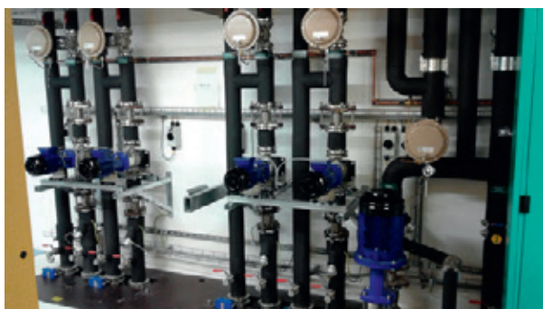
Fig. 5.3.2.1: Picture of cooling station KKV14 installed at SwissFEL.
