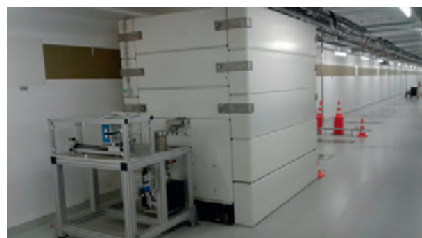
Fig. 5.2.1: Top picture: Installation of the beam dump shielding blocks in the beam dump groove (2013). Bottom picture: Athos beam stopper in front of the undulator line.
