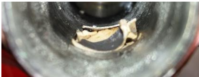
Figure 3-13 Duralco 128 epoxy, degraded from prolonged exposure to hot steam
