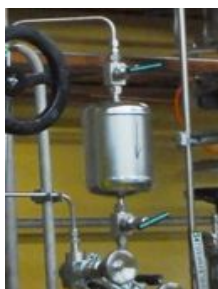
Fig. 1: Filter device installed in the SINQ cooling workshop.
