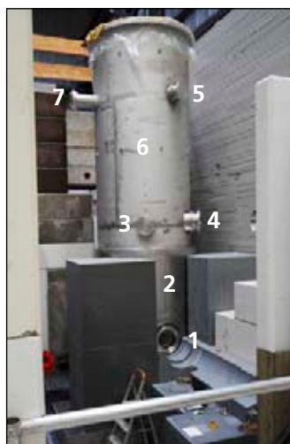
Figure 1: UCN tank system in the half-assembled iron radiation shielding.
