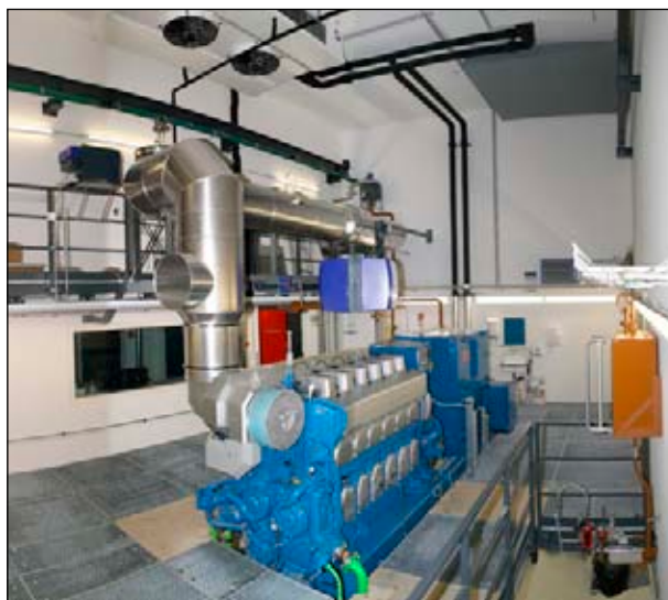
Figure 2: Panoramic view of the 1.2 MW 6-cylinder engine at the Large-Engine Test Facility.
