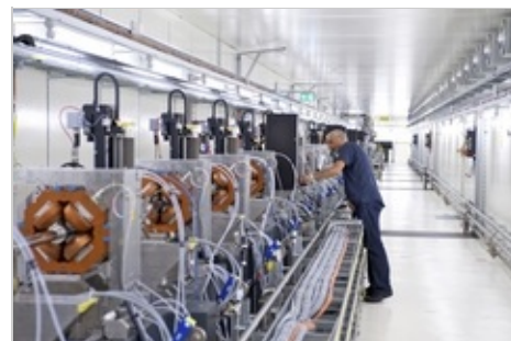
View along the tunnel of the 250 MeV injector. Technologies are being tested here for the first part of the SwissFEL accelerator. As soon as the final SwissFEL buildings are ready, the facility will be installed in them and will comprise the first section of SwissFEL. (Paul Scherrer Institut/Frank Reiser)
